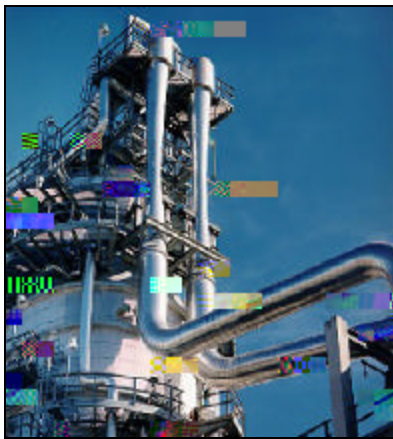
Figure 7. First stage ejectors for CVDU.
